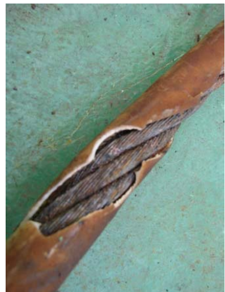
Figure 2. Corrosion beneath plastic sheathing.
